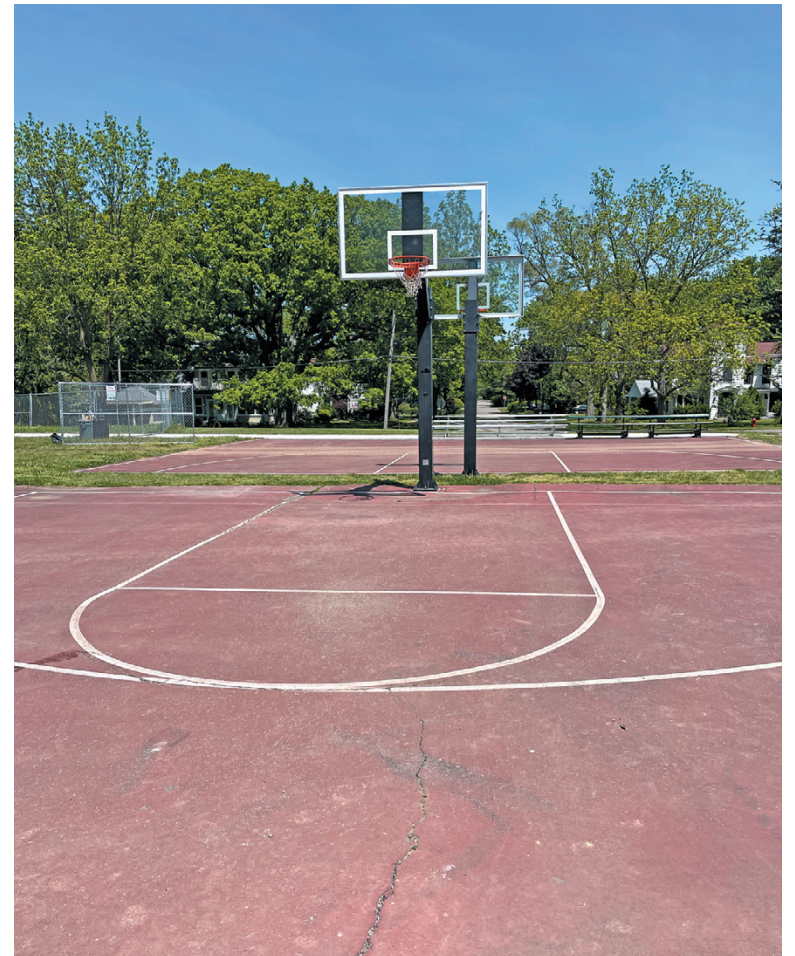
Village of Lewiston trustees voted to replace the cracked basketball court pavement, contingent upon receiving funds from a pending property sale.
